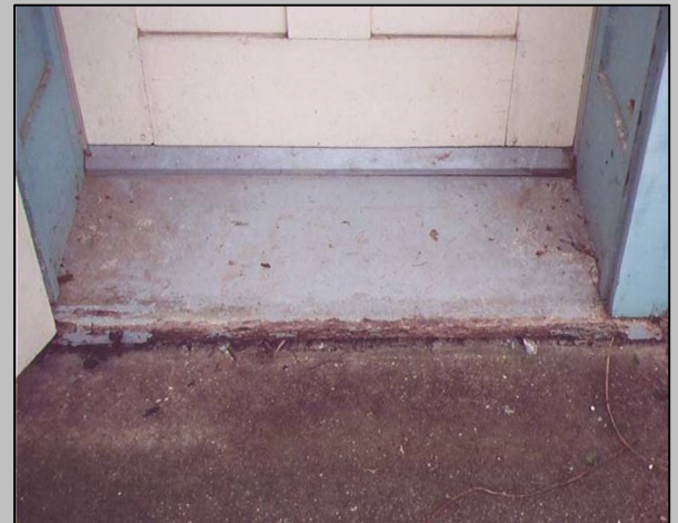
Door components are especially susceptible to deterioration from constant exposure to weather and foot traffic. Elements such as thresholds and the bottom of frames are particularly vulnerable.
