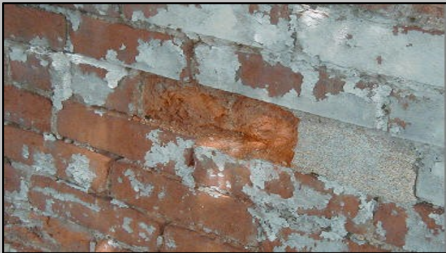
Never sandblast or use high-pressure power washing to clean masonry. Doing so can compromise the building structure by scarring masonry surfaces beyond repair, which will allow excessive moisture into the masonry.
