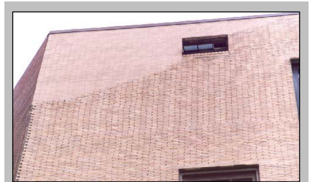
When masonry is repaired or replaced, new materials should match the existing historic materials. Failing to match materials can severely detract from the visual aesthetic of the building.
