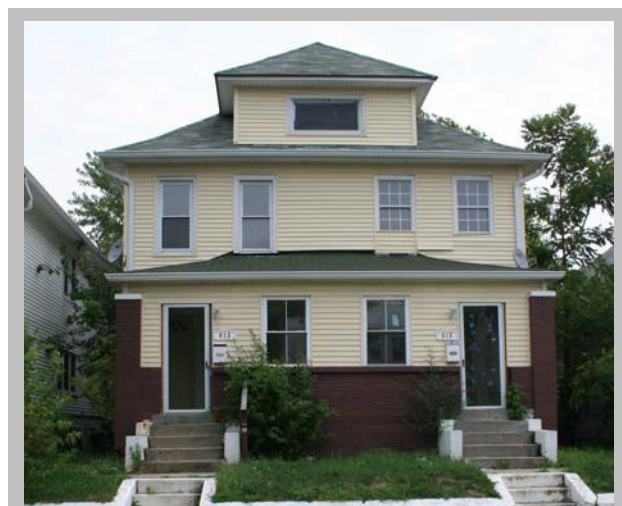
When replacing windows, you should always choose a replacement that matches the historic characteristics of the original. Failing to do so, as in this rehabilitation example, can compromise the aesthetic of the house.
