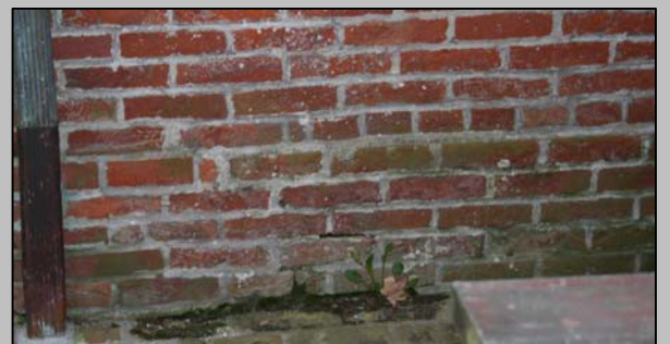
Moisture is the most significant cause of decay in masonry. Seen here are examples of spalling, efflorescence, and organic growth, all caused by excessive moisture.
