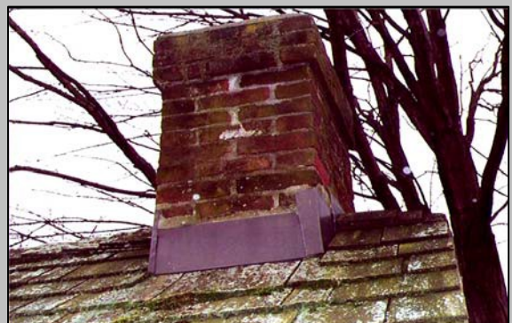
Deterioration that is not addressed can compromise the effectiveness and soundness of your roof system.
